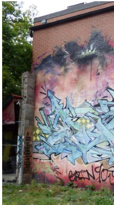
29. The west side of the south elevation; note the mix of brick masonry and cinder block infilling, in addition to the remnants of a connecting wall to the former building at 23 St. Andrew Street (Source: ERA Architects).
