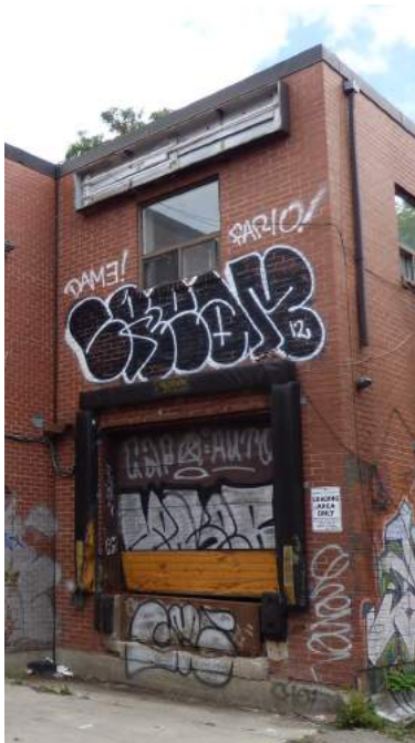
28. Photo showing the poor/damaged condition of the masonry and concrete sill at the loading door at the west elevation (Source: ERA Architects).
