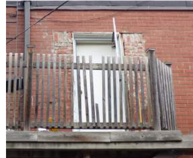
26. Window opening at the west elevation that was converted to a door. Note the poor condition of the brick surround (Source: ERA Architects).
